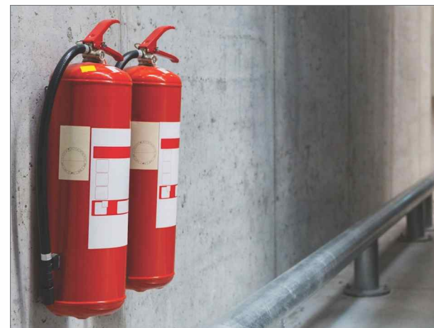
▲ Fire Fighting Systems
